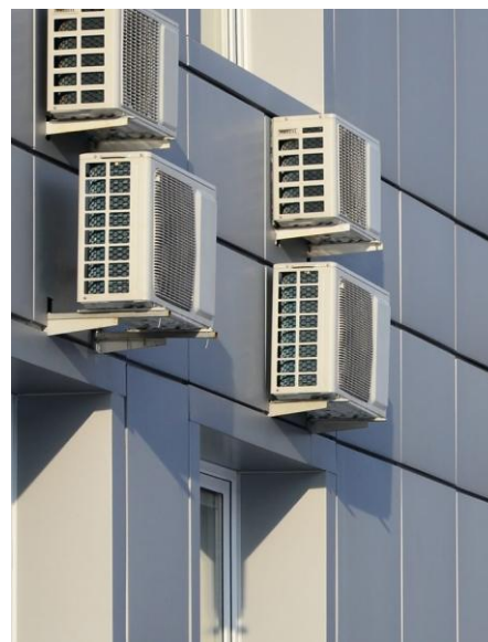
Figure H1b: Air-source heat pumps installed on a building.
